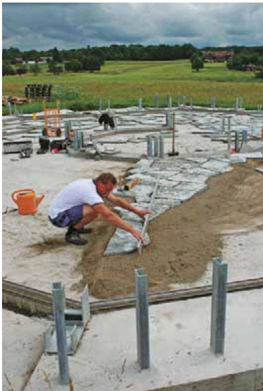
Local entrepreneur installing BIRD Project investment using traditional material Photo: Jan Lundegrén
