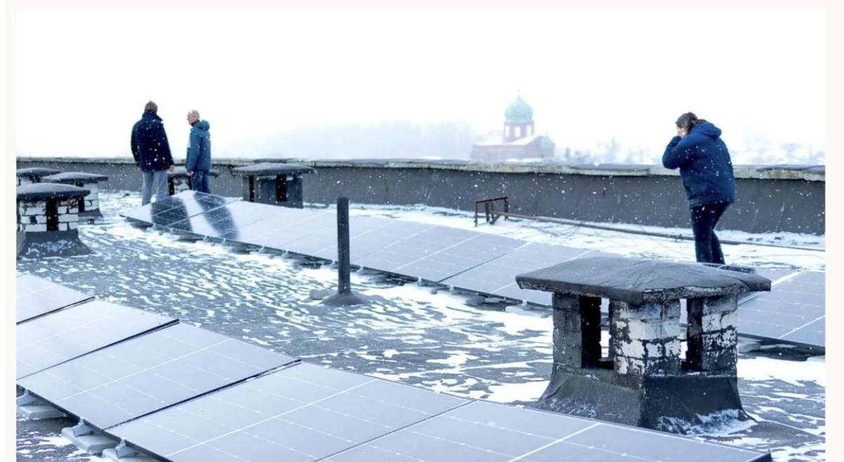
Recently installed solar panels atop Koriukivka Central Regional Hospital in Koriukivka, Ukraine. COURTESY OF ENERGY ACT FOR UKRAINE FOUNDATION
